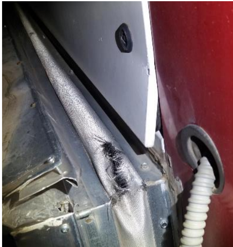
Ventilo-convector corrosie leidingen EGL
